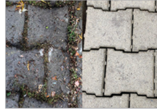
The PaveDrain block system, before and after maintenance.
